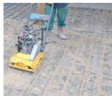
Photo 83 - Damage des joints.
